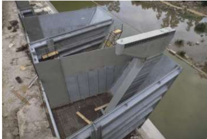
Fig.13 Retaining structure of the "Hydroplus" type
