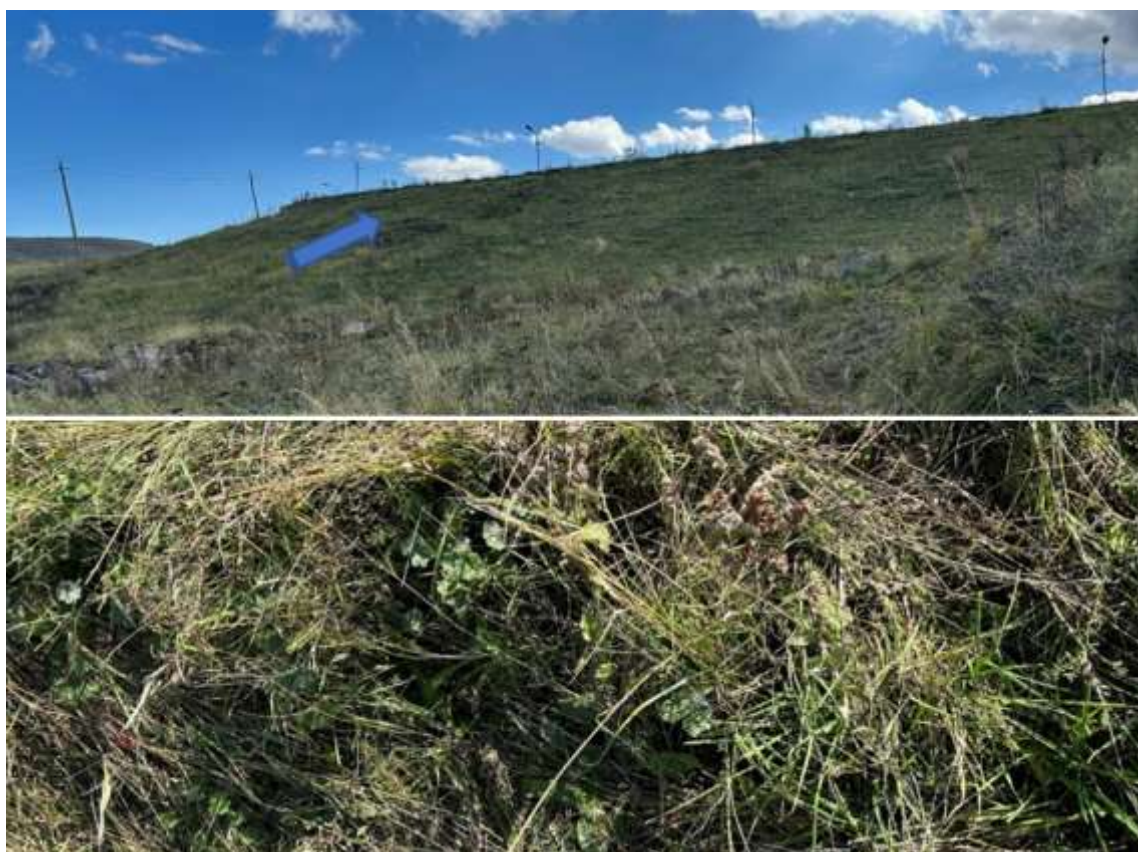
Fig. 6 Landslides in the lower slope of the Gegharkunik 2 reservoir dam after the appearance of a ravine in 2020
