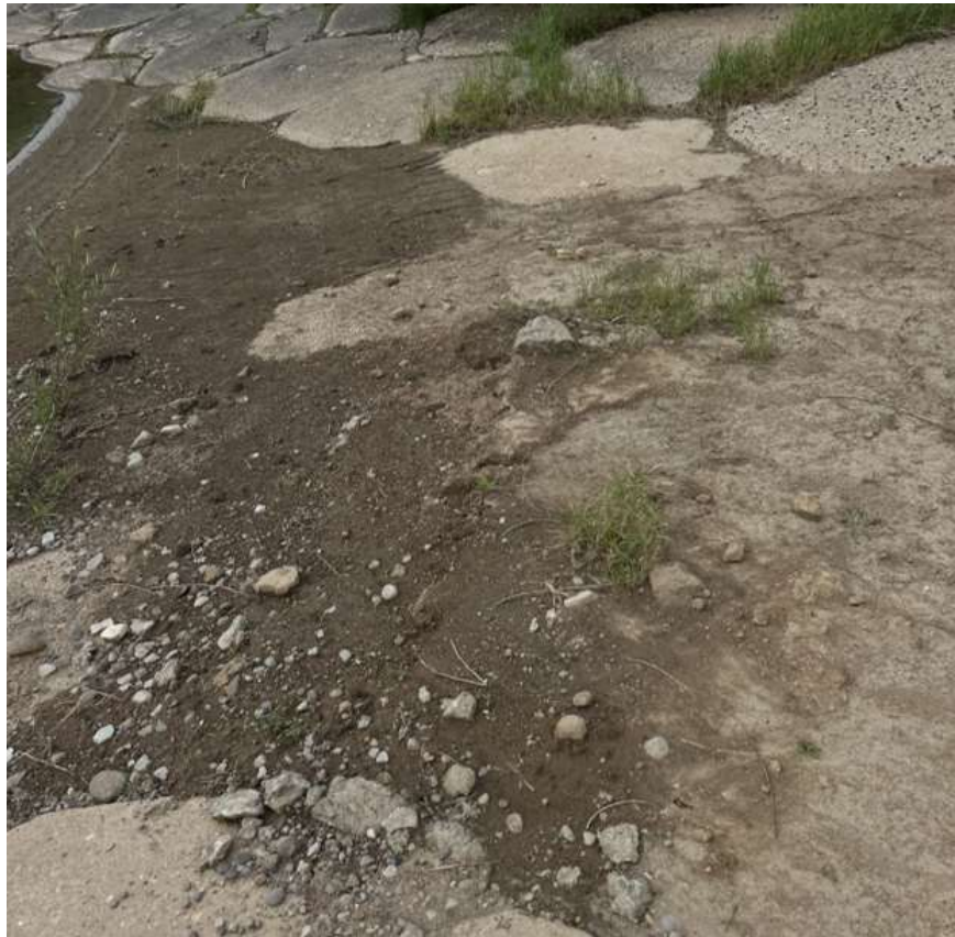
Fig. 2 Washouts on the dam body
