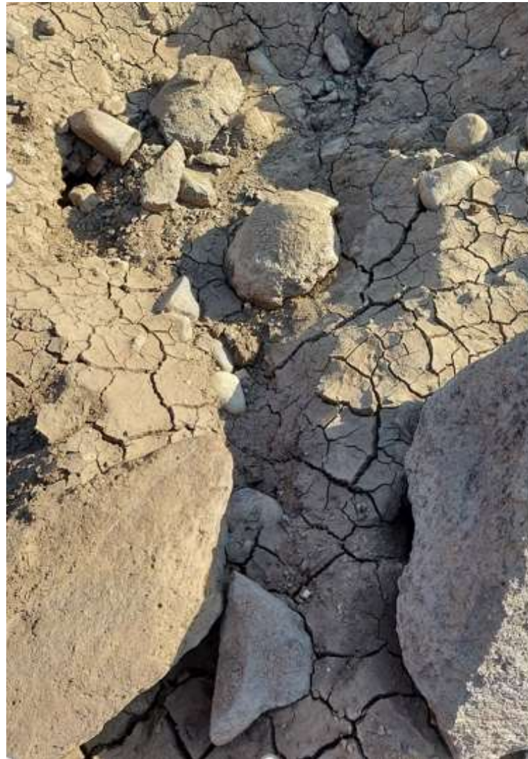
Fig.2. Washouts on the dam body
