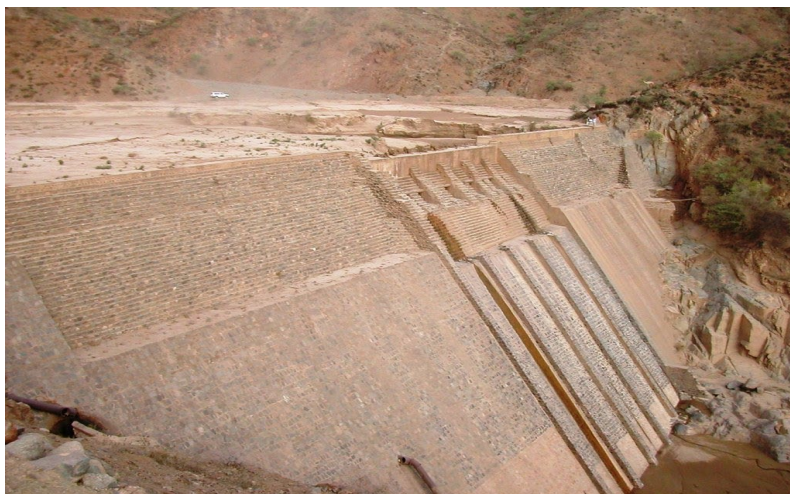
Fig. 1 Denata reservoir in Eritrea completely filled up with sediments (North-Eastern Africa) Photo by Adriano de Vito (Google Maps)
