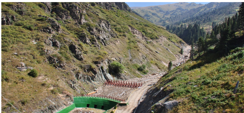
Fig. 1 Cascade of mudflow protection facilities: downside monolithic – made of reinforced concrete, upside– made of collected metal constructions.
