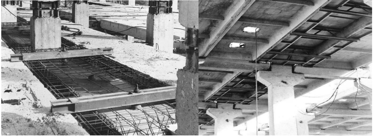
Figure 1. Metallic suspended block-form for monolithic reinforced concrete beams of multistorey industrial buildings a) top view, b) bottom view
